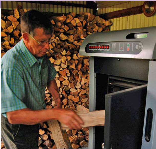
Wood powered heating system
