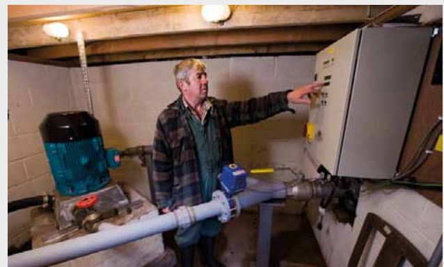
Inside a turbine house
