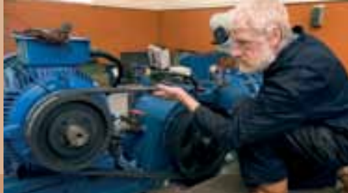
Hydroelectric turbine, Talybont Reservoir
